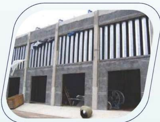
Argo PANTES PROJECT - Intake Sound Attenuators MM 2100 Cibitung - Bekasi
